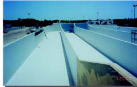
F R P Lining for Concrete Tank
