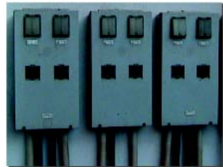
Two Customer Meter Boxes
