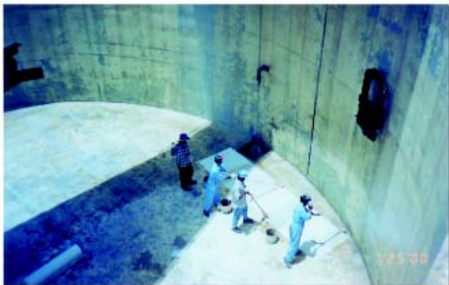
F R P Lining for Effluent Tank
