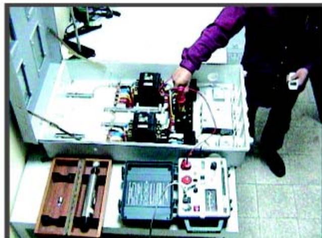
High Voltage Testing Unit
